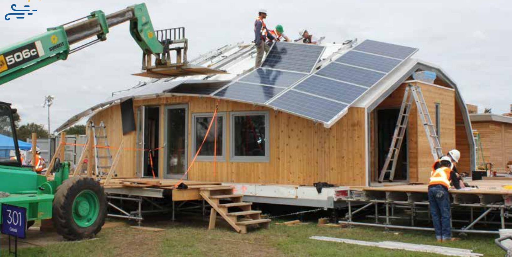
Installing solar panels on the roof of a Traditional Living house at the University of Calgary. Photo: Carol Anna/U.S. Department of Energy
